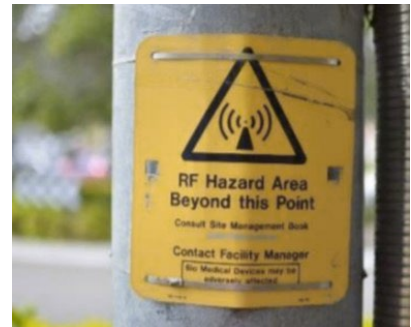
Example of identifier plate located near an RF transmitter
