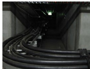
Cable terminations and pits
