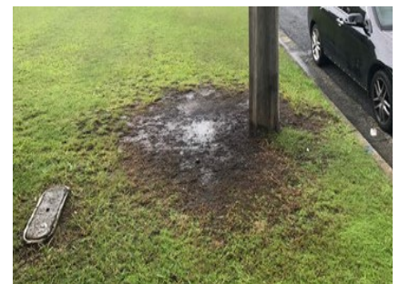
Contamination from a leaking pole transformer
