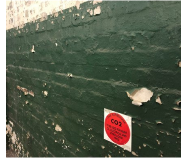
Lead paint on substation wall
