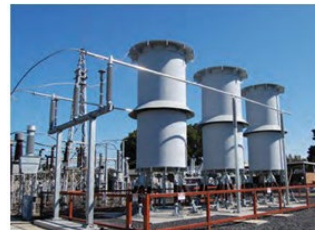
Air cored reactors
