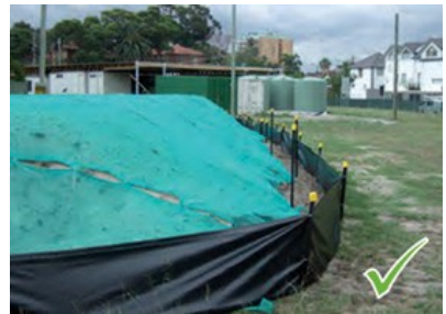
Stockpile covered to prevent dust and a sediment fence used to filter run-off
