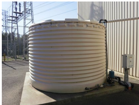
Washbays using recycled water are generally exempt from water restrictions and water saving rules
