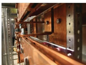
Low voltage busbars
