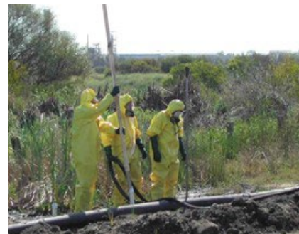
Working in contaminated areas may require special PPE
