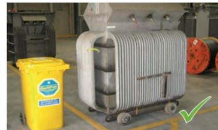
Spill kits should be readily available near oil storage areas
