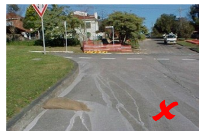
Saw-cutting slurry has not been contained effectively
