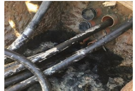
Unknown material seeping into trench will need to be assessed
