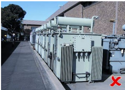
Equipment stored too close to the bund wall means leaks may not be contained
